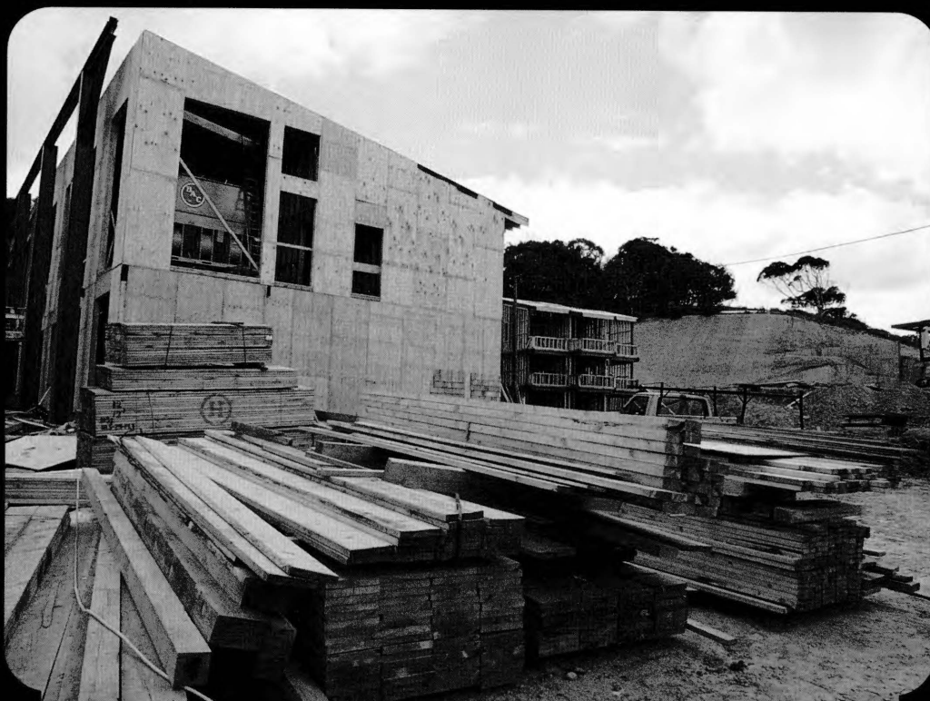
The W. M. Keck Foundation Center for Ocean Atmosphere Research under construction at Scripps
