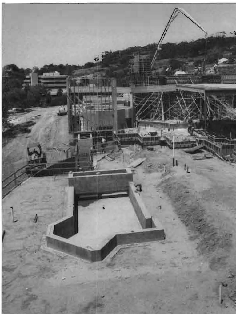
Tide pool exhibit foundations are poured, construction of the Stephen Birch Aquarium-Museum in background.
