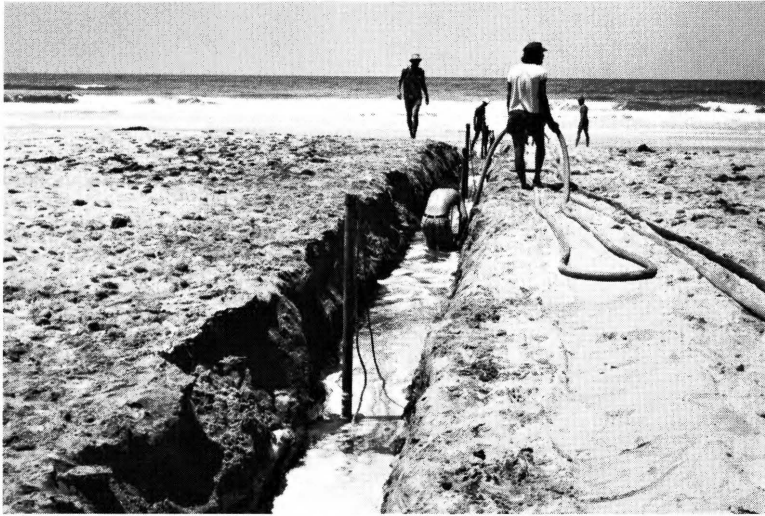
Duct-flow fluidization cuts inlet channel across beach as part of Sea Grant research project carried out by members of Shore Processes Study Group at Los Peñasquitos Lagoon, San Diego.
