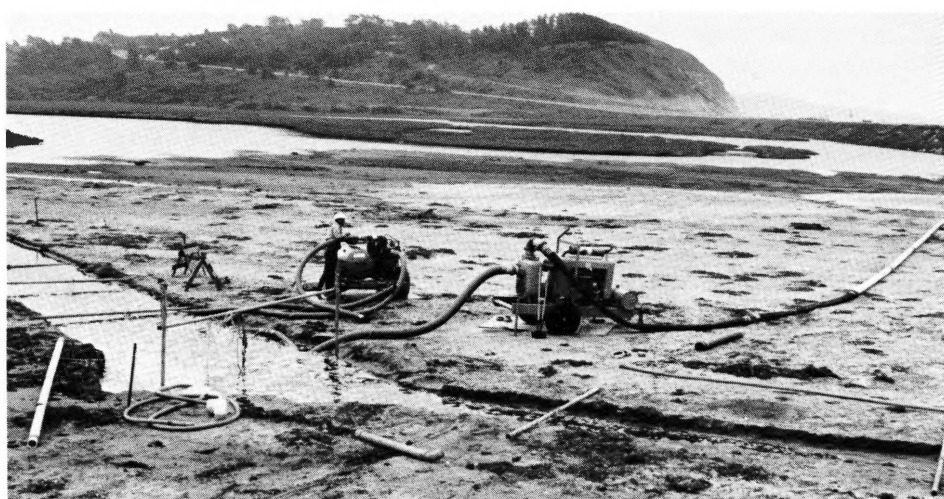
Pumping equipment used in feasibility study of duct-flow fluidization as method of fluidizing and maintaining a stable lagoon entrance channel to Los Peñasquitos Lagoon in San Diego County. Work was part of a Sea Grant research project carried out by Dr. Douglas L. Inman and Charles E. Nordstrom, of the Shore Processes Study Group.
