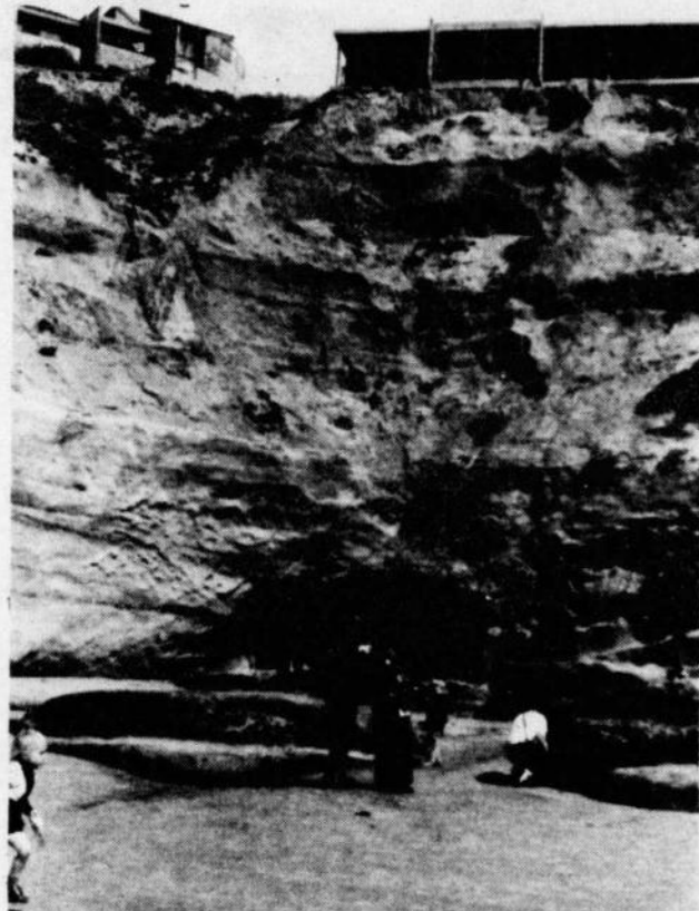
Cave in base of bluffs caused by tides
