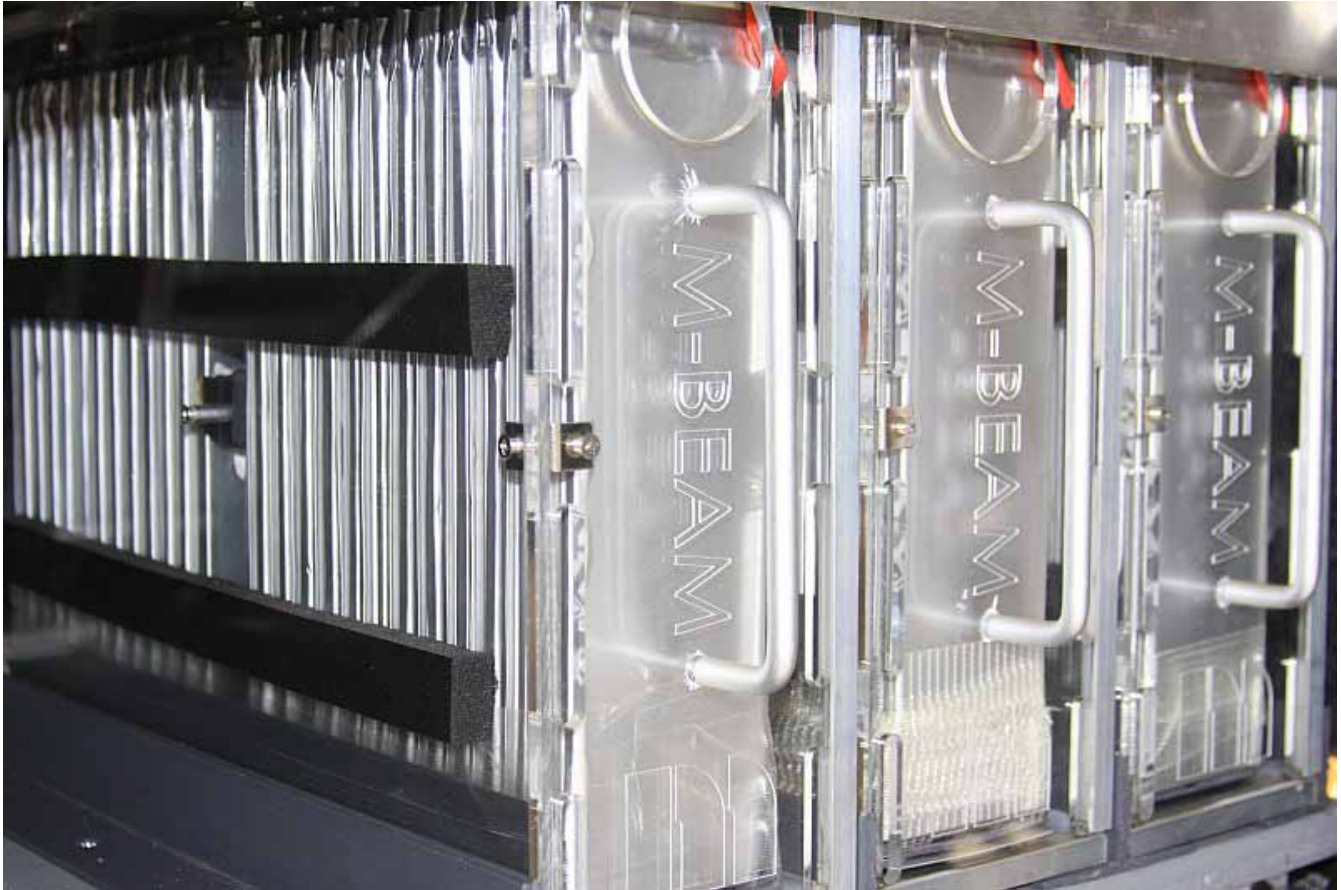
Close-up of the battery modules
