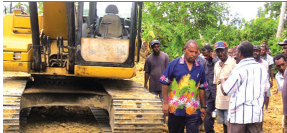
Minista Richard Maru i toktok wantaim ol pipel long seremoni bilong brukim graun long wokim rot projek.
