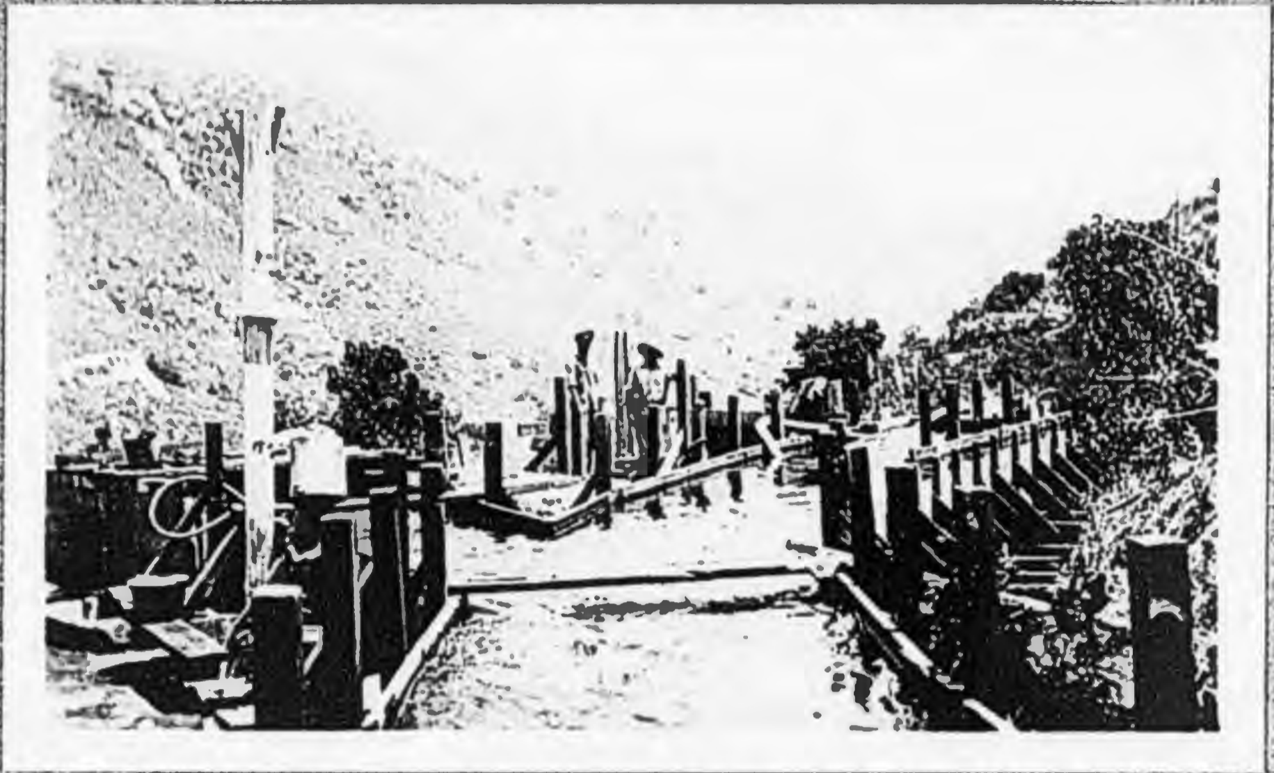
Junction of Main Flume, South Fork Siphon, and South Fork Feeder after Repairs.
