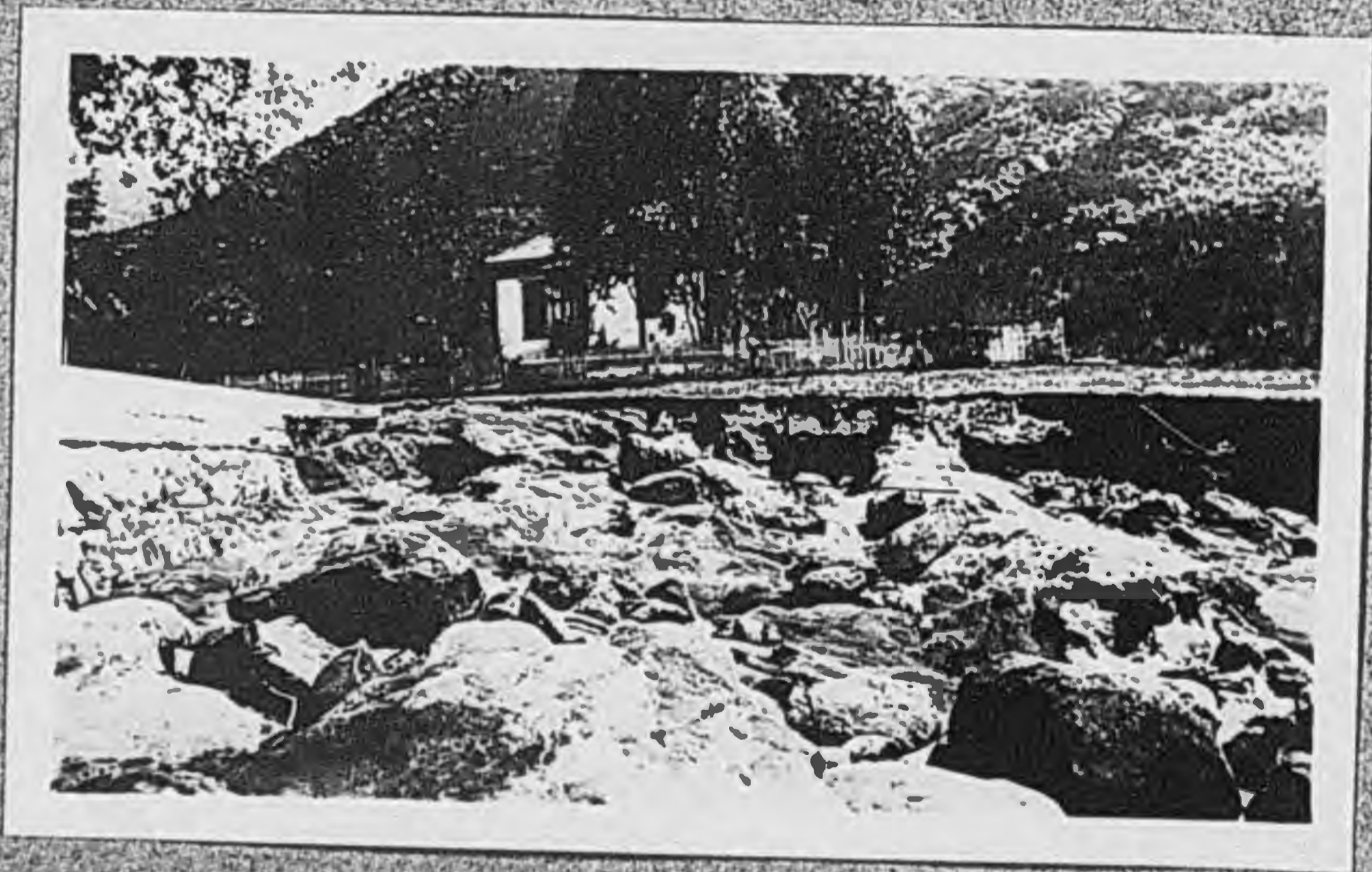
Shows Erosion of Material Below Dam and Undermining of East Wing Wall.
