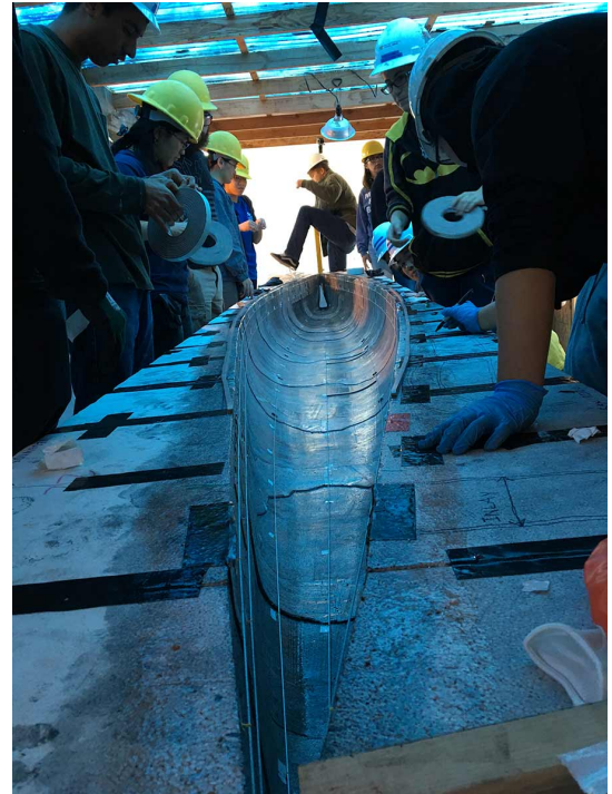
Students spend nine continuous hours on Pour Day placing alternating layers of concrete and mesh for support around their canoe mold.
