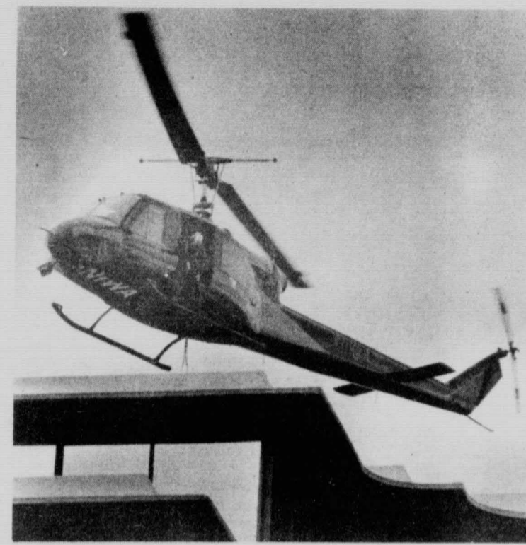
Central library received several new air conditioning units early Sunday morning. Due to their bulk, the units were air lifted into place using a special sling rig mounted on a helicopter.
