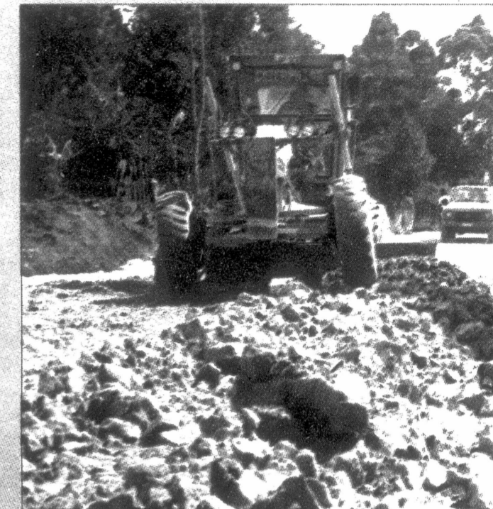
Road maintenance and up-grading has been allocated more funding in all the districts.
