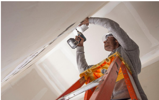
UC San Diego structural engineering graduate student Srikar Gunisetty installs a sensor in the building.
