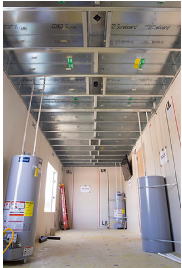
Several water heaters also have been placed on the sixth floor.
