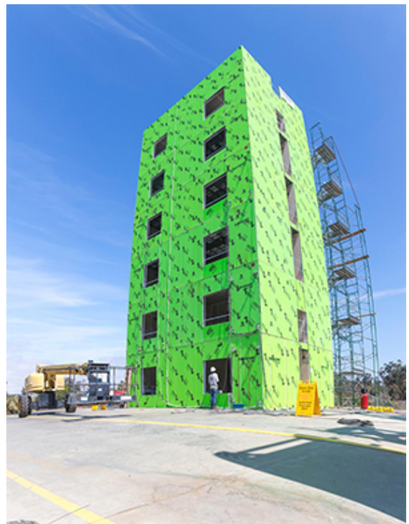
Researchers will test a six-story cold-formed steel framed building. Photos from current project on Flickr
