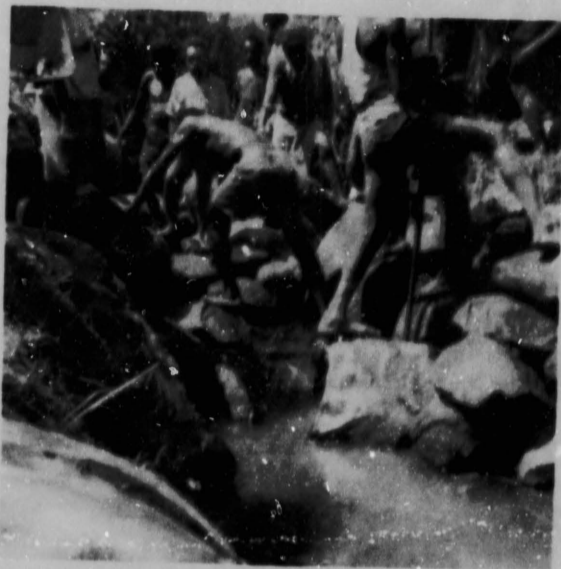
A creek on the Kaintiba road and workers selecting stones to rearrange into a culvet.
