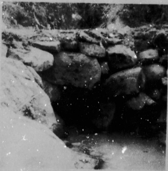
The same creek after the culvet has been constructed. Note that this picture was taken from the same position as the one above with the same rock and the same blade of grass in the foreground.
