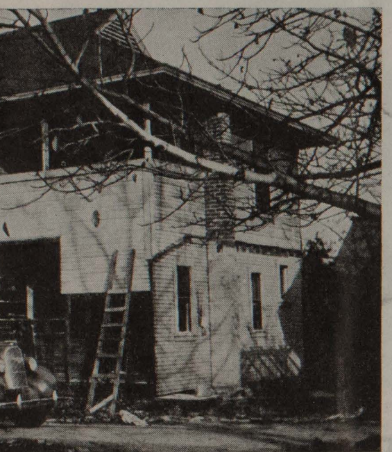
The second home of the Waite family in process of demolition to make way for more modern place of abode.
