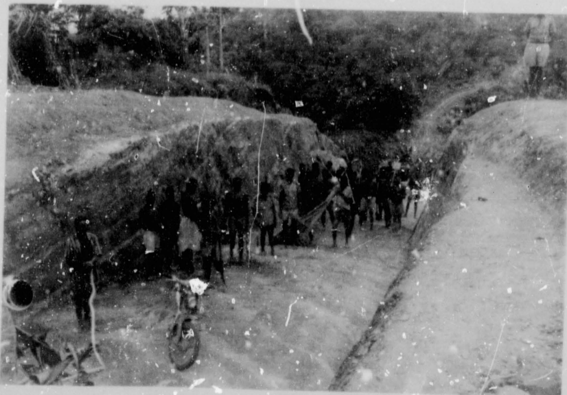
Another sandstone box cutting which lowered the final grade of the section shown from 17% to 9% over the length of the work.
