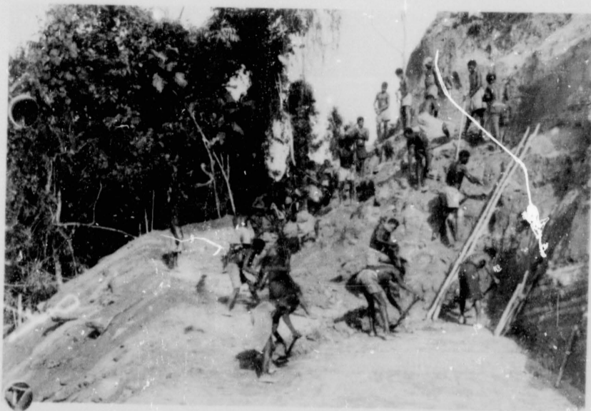
Recutting a sandstone ridge; this section within the picture was completely removed.
