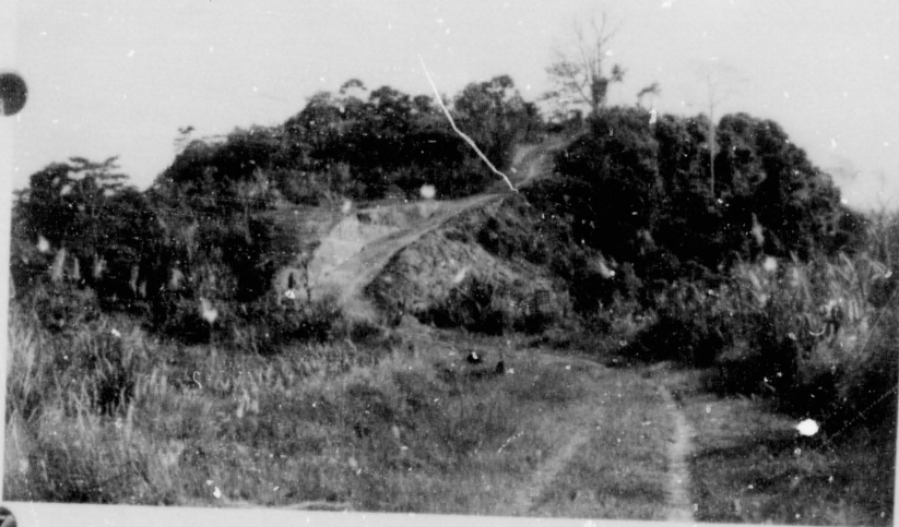
Two recut sections, both about 250 ft. long. The lower is sandstone, max. cut 10 ft. Over all grade is now 3%; before it varied between 17 and 4%
