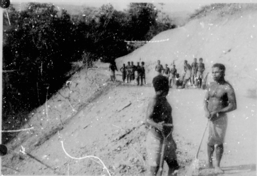
Bench cut in soapstone material. Note steep battering of cut. The old road followed the top of the bank to the right. Max. cut here is 16 ft. while this cut was 430 ft. long.
