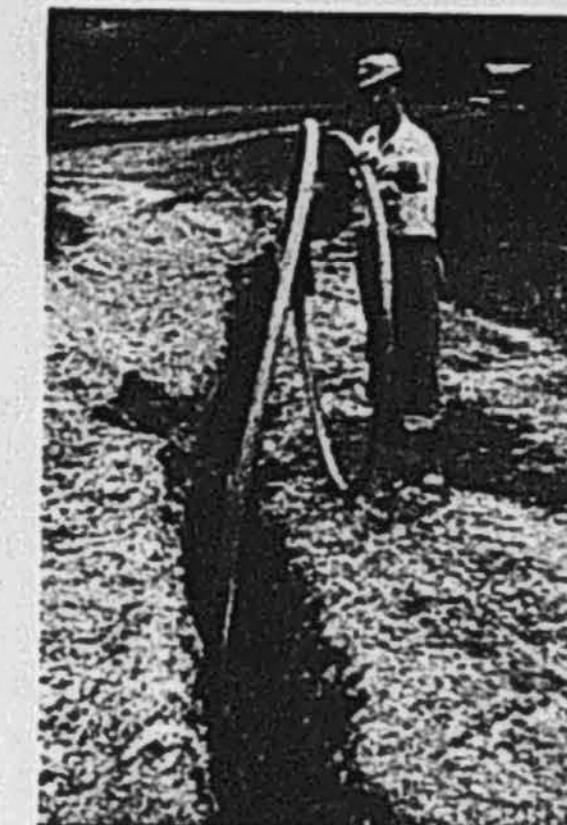
Exact line and grade were not necessary with this flexible plastic pipe.
