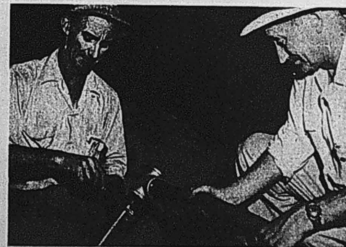
Special, hard plastic adapters, threaded at one end, make the connections. The adapter's free end is squeezed into pipe and locked with a freeze-type coupling.
