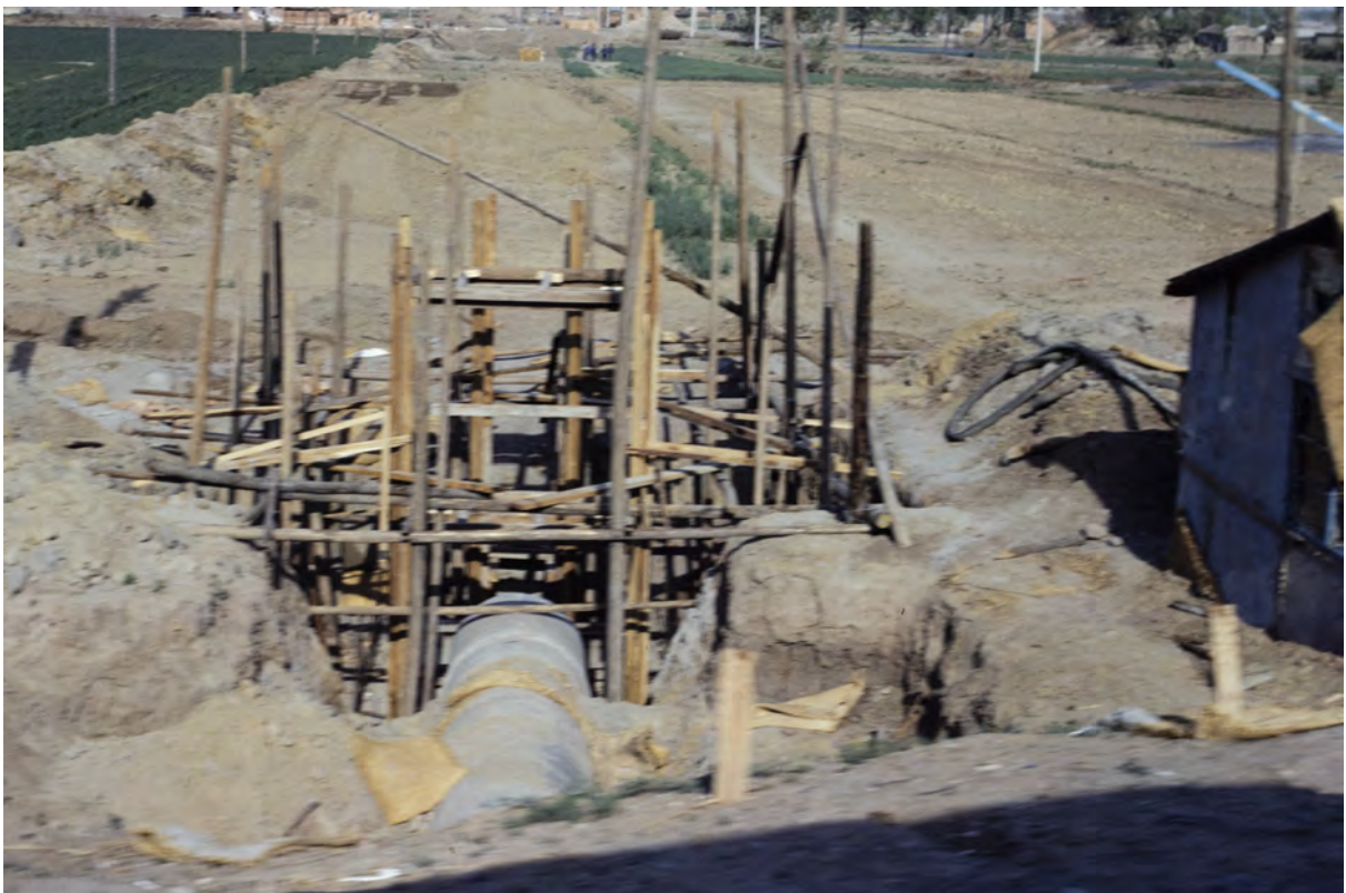
Irrigation pipes building
