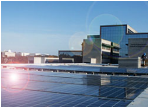
UC San Diego has photovoltaic panels on rooftops and parking
