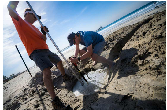
Researchers with the Center for Climate Change Impacts and Adaptation at Scripps install pressure sensors in the sand in Imperial Beach on Nov. 13, 2018. These sensors will assess the wave run-up predictions in flood-prone areas. Photo by Erik Jepsen/UC San Diego Publications
