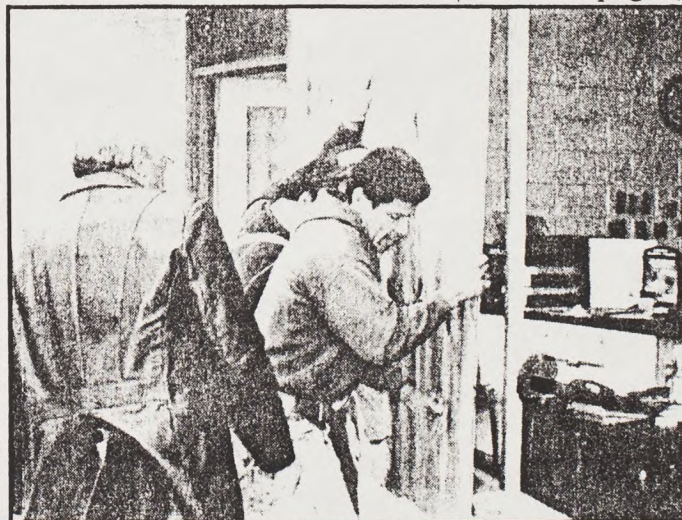
Ray Gonzales with the help of Luis Natividad (partially hidden) and under the supervision of Richard Resendez board up the front windows of the shop.
