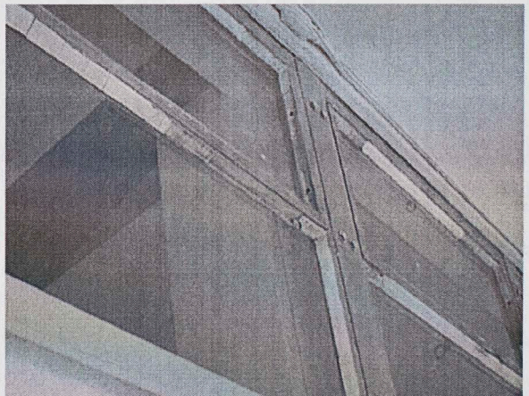
Wooden window frames are deteriorating and need to be updated with modern metal frames.
