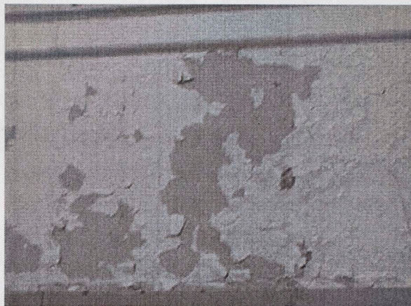
Paint will not adhere long on moisture-damaged exterior walls.
