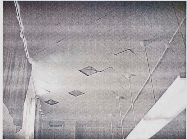
Ceiling tiles are coming loose due to age.
