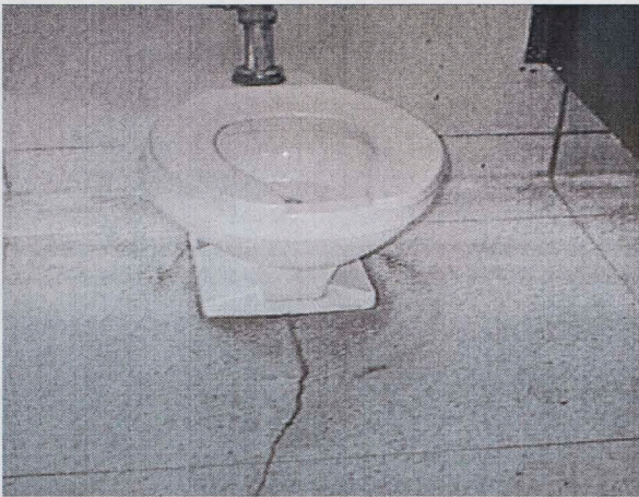
Old leaky fixtures have been replaced, but not before water penetrated the flooring.
