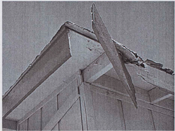
Dry rot and roof leaks have caused permanent damage.
