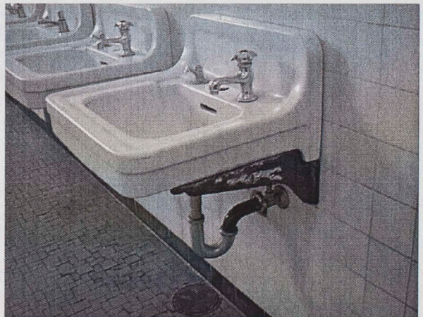
Rusting sink brackets need to be replaced.
