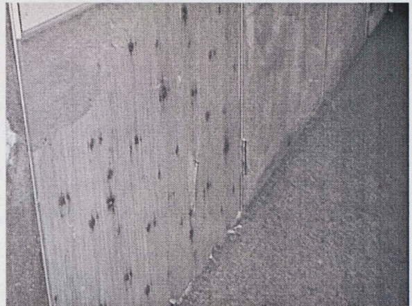
Vinyl coating that covers classroom wall has deteriorated and fallen off.
