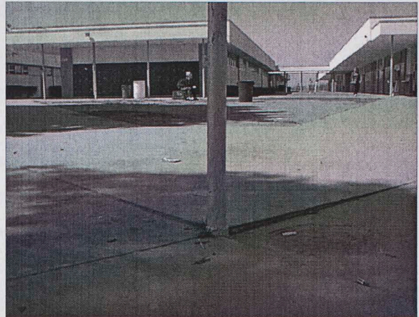
Ground settlement has made student walkways unsafe in places.
