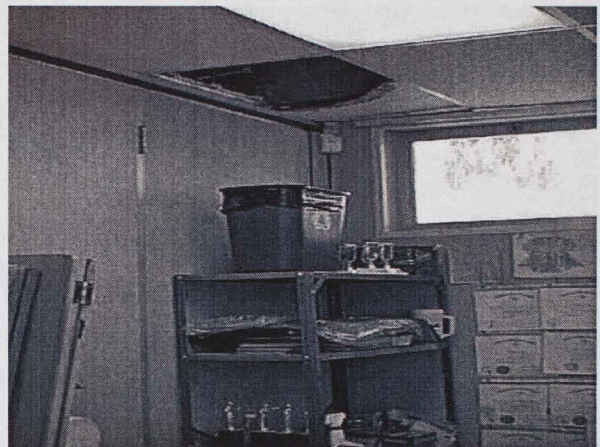
Roof leaks into classroom from above the ceiling.
