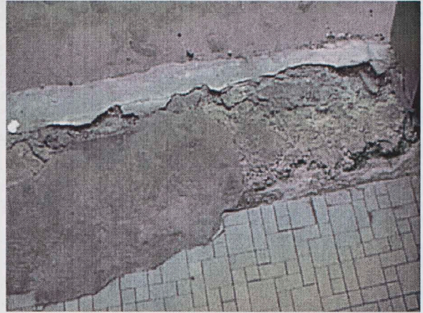
Water leaks in the bathroom have caused permanent floor damage that can only be patched until replaced.
