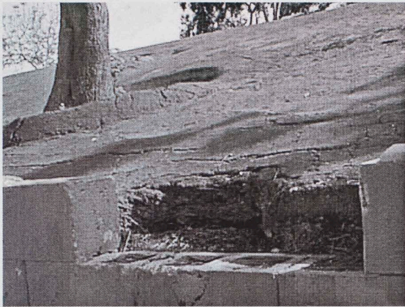
Water has penetrated the hardscape and eroded a retaining wall adjacent to student walkways.
