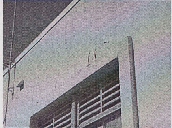
Exterior walls are painted regularly, but water damage and age limit the positive benefits.
