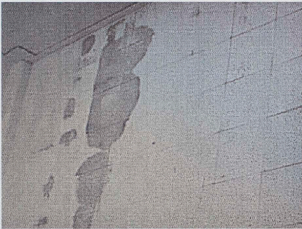
Wall tiles have fallen off due to roof leaks above.
