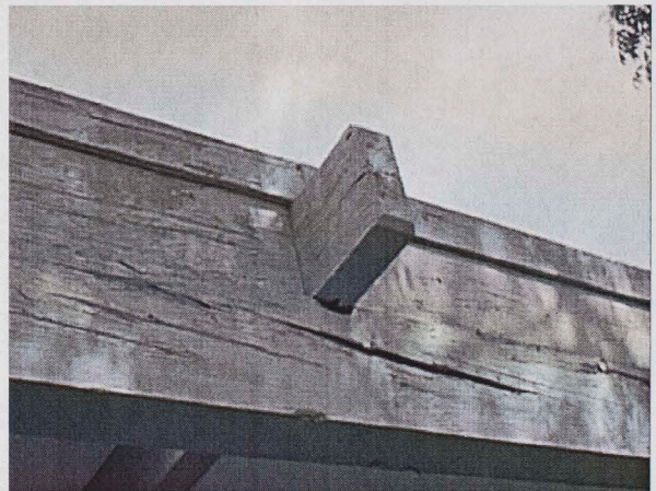
Dry rot has invaded aging support beams.
