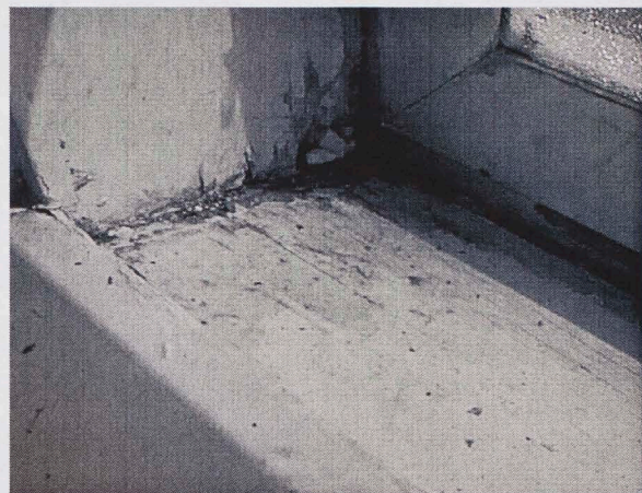
Interior wood window frames are deteriorating due to age.
