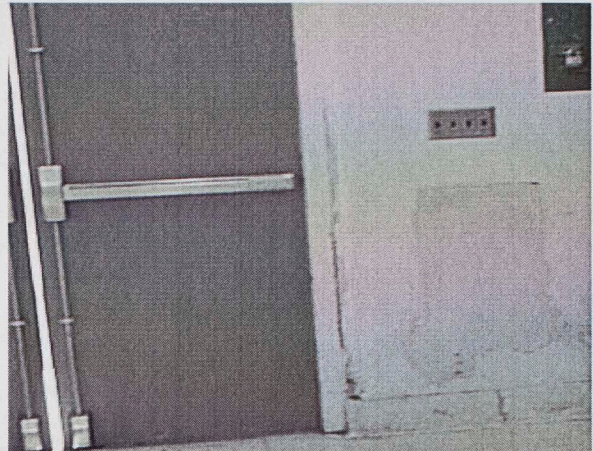
Because moisture has penetrated the wall and door frame, repeated patches and paint only mask the problem.
