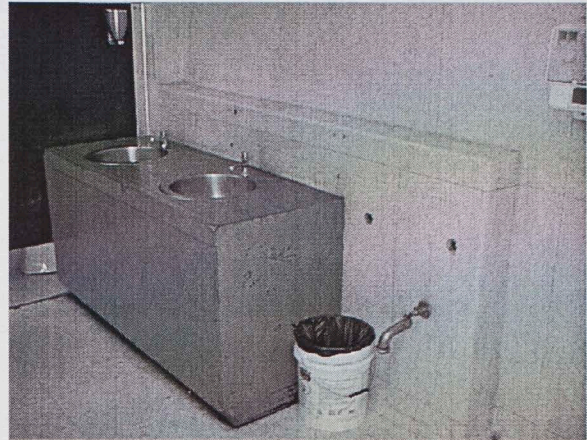
Wooden sink cabinets are rotting from moisture.
