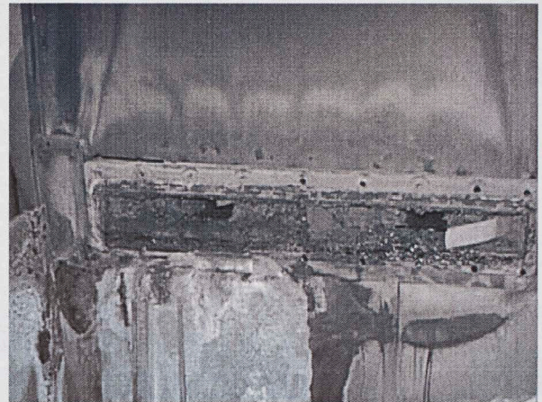
Boiler shows signs of disintegration from age.
