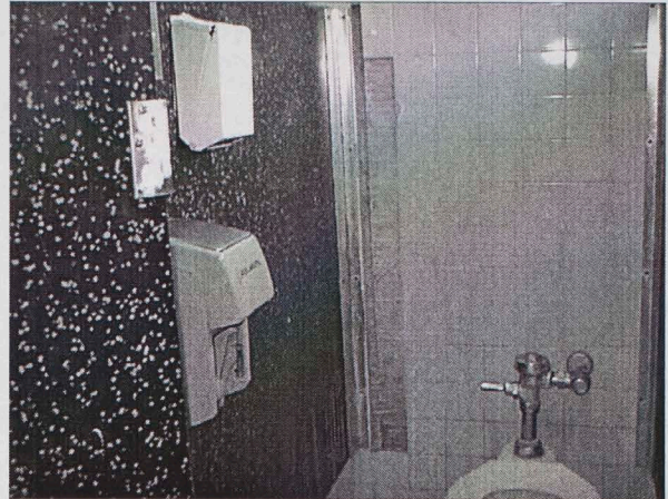
Tile on bathroom walls is coming off due to age.
