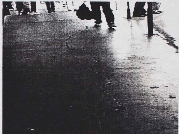
Cracked walkway is visible from uneven soil settlement.
