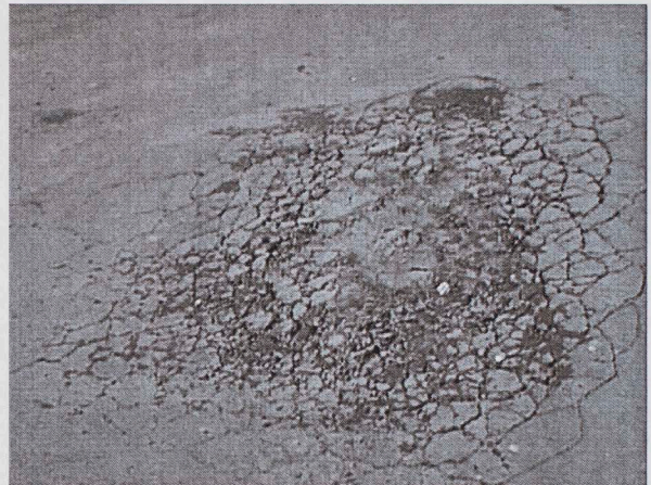
Ground water and uneven site conditions have damaged student walkways.
