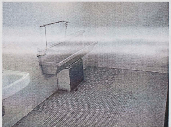
Old metal urinal is deteriorating and needs to be replaced.
