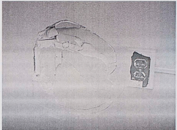
Wall materials crumble from moisture penetrating the wall.
